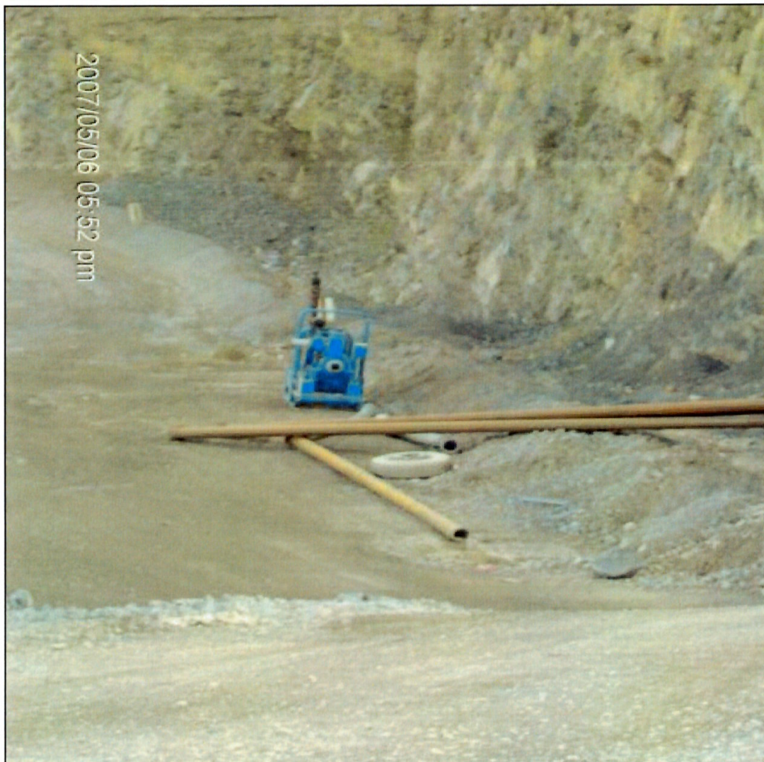
Water pump and pipes on quarry floor.
