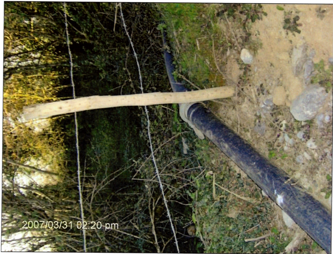
Water pipe leading onto channel beside canal bank
